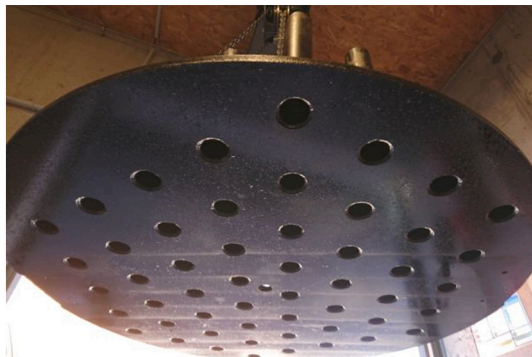
Fig. 3. HTF distributor at the top of the tank.
